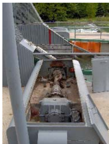
Installed at Site
