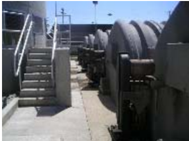
Rotating Biological Contactor (RBC's)
